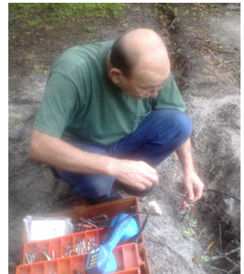
Bart (AF4TK) and broken cable
